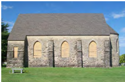
Marysville Cemetery Chapel. Marysville, Marshall County, Kansas. East Elevation. Photo by William E. Fischer, Jr., 9/1/2014
