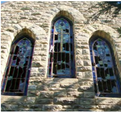
Marysville Cemetery Chapel. Marysville, Marshall County, Kansas. South Elevation Windows Over Entrance. Photo by William E. Fischer, Jr., 9/1/2014
