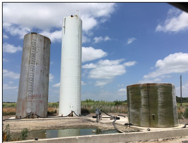
Photo 4. Standpipes with Ground Tank at right
