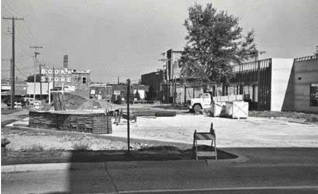
1987 construction of commercial center at 14 th Street and Anderson Avenue (KSU Morse Department of Special Collections).
