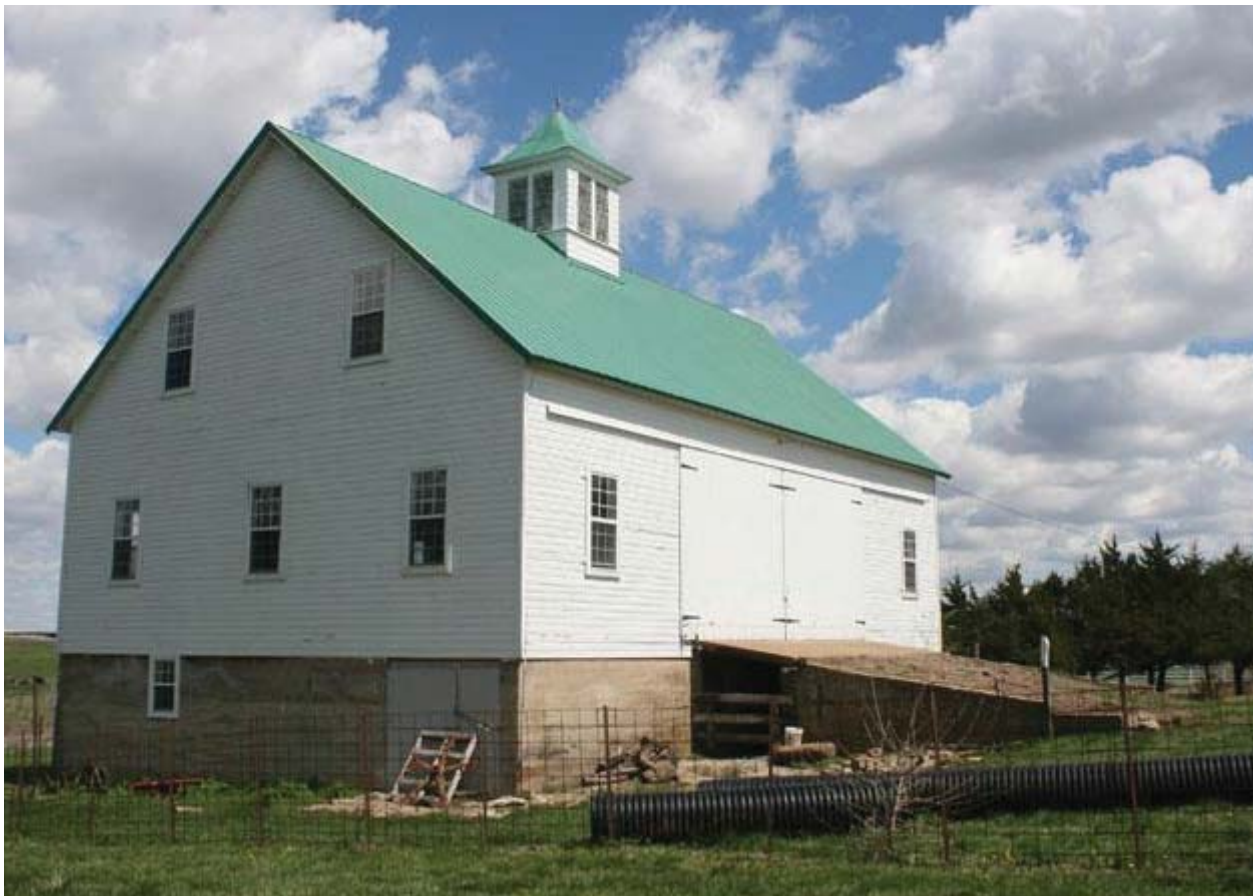
The Churchbaugh Barn was constructed ca. 1920, when farmers were flush with cash following World War I. KHRI. Photo by Susan Ford.
