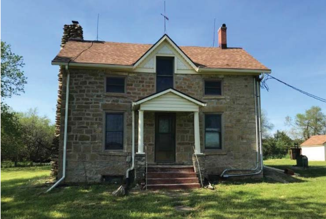
The McQuillion House was built as early as 1856 when Thomas McQuillion first settled in Willow Springs Township. The centered gable, reminiscent of vernacular Gothic Revival houses, was likely added in ca. 1870. Photo by Christy Davis.
