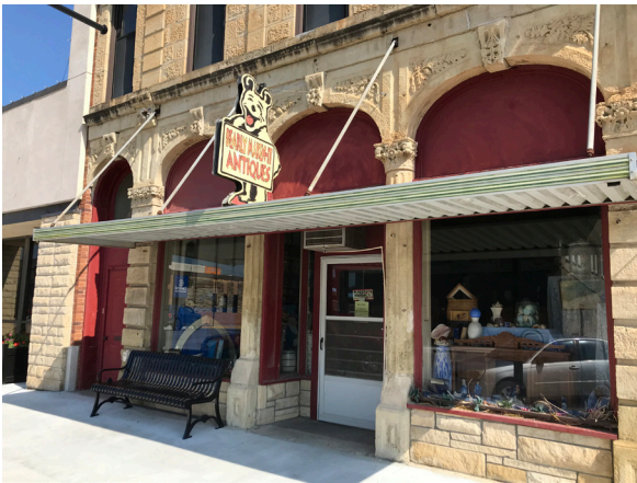
Italianate Storefront at 308 E Main partially modified
