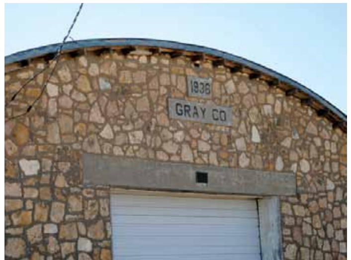
The Gray County Shops in Cimarron were built by the Works Progress Administration in 1936. Photo courtesy Christy Davis.
