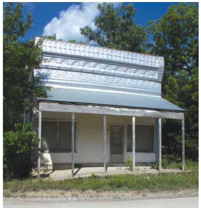
One-story front by Mesker Brothers Iron Works with stamped brick siding panels on side elevations. Clements, Chase County.
