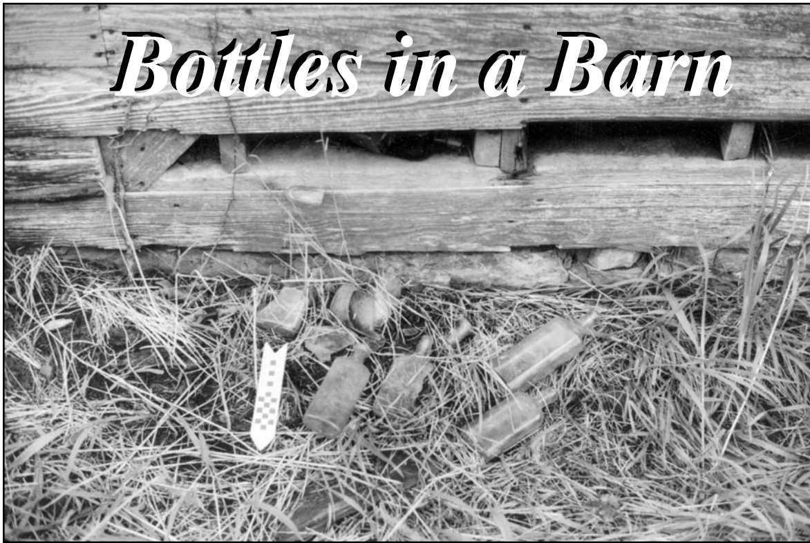
What at first glance appeared to be a pile of glass turned out to be numerous bottles falling out of the wall cavity of the barn where they had been stashed.
