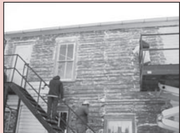
Work is currently underway at the Constitution Hall State Historic Site in Lecompton.
