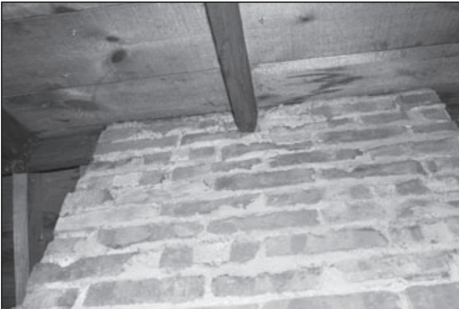
Chimneys can be a source of air leaks.
