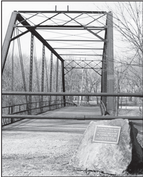
The Elk Falls Pratt Truss Bridge is shown after preservation work made possible by $9,546 in Transportation Enhancement funds. The bridge crosses the Elk River in Elk County.
