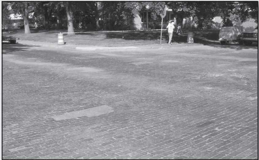
Transportation Enhancement funds have assisted with restoration of brick streets in Emporia, Goodland, and Troy.
