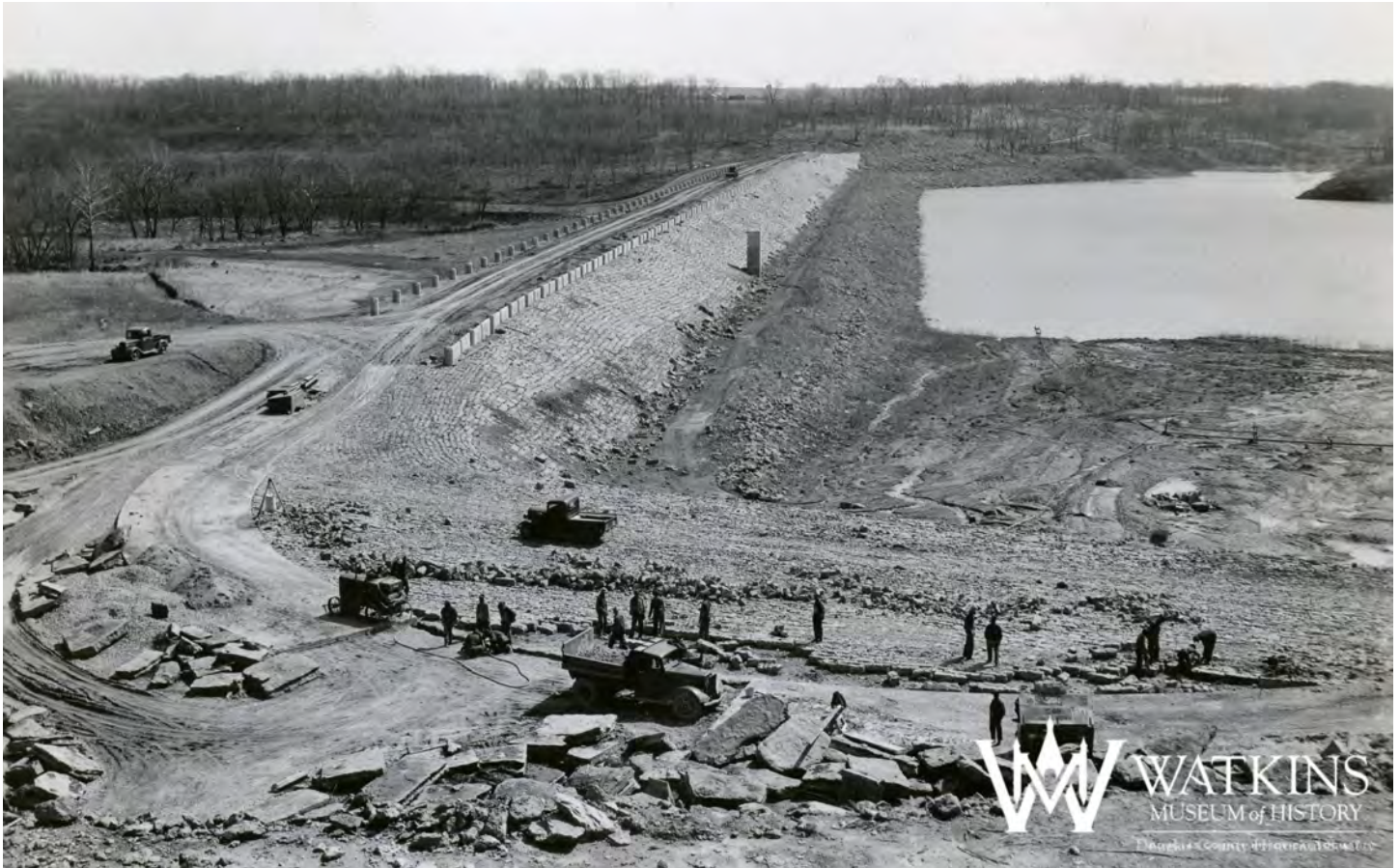
Figure 11: Historic Photo of Lone Star Lake Dam under Construction, looking east. Unknown Date. Image provided by the Watkins Museum of History
