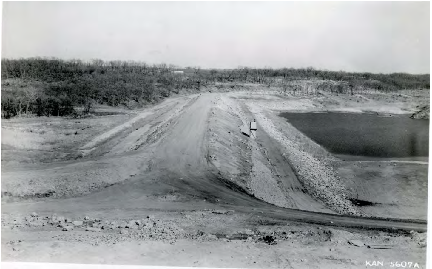
Figure 8: Historic Photo of Lone Star Lake Dam under Construction, looking east. Unknown Date. Image provided by the Watkins Museum of History.
