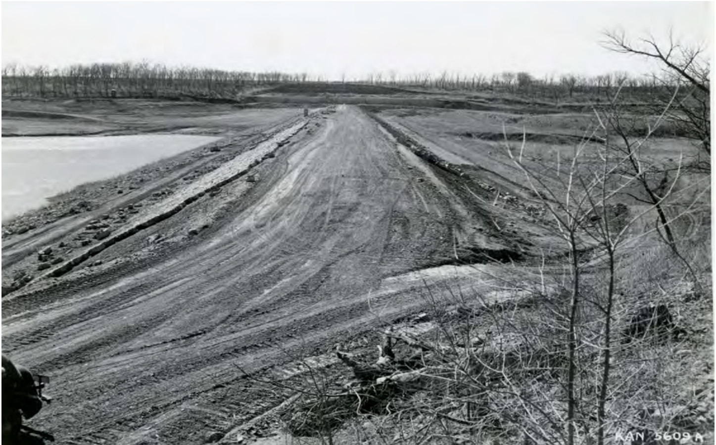
Figure 9: Historic Photo of Lone Star Lake Dam under Construction, looking west. Unknown Date. Image provided by the Watkins Museum of History.
