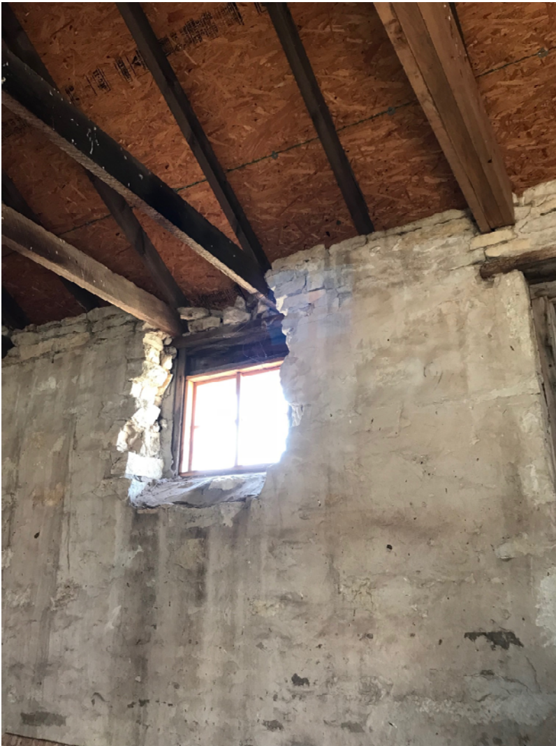
Figure 9: Small fixed window in Limestone Outbuilding, structural repairs to trusses and new plywood roof sheathing.
